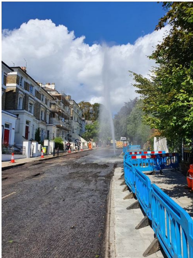
More burst pipes, August 2020
