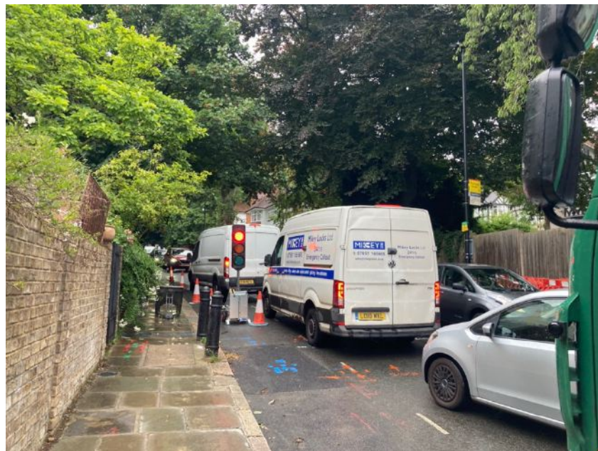
Further traffic jams resulting from work on pipes and temporary traffic lights, August 2024
